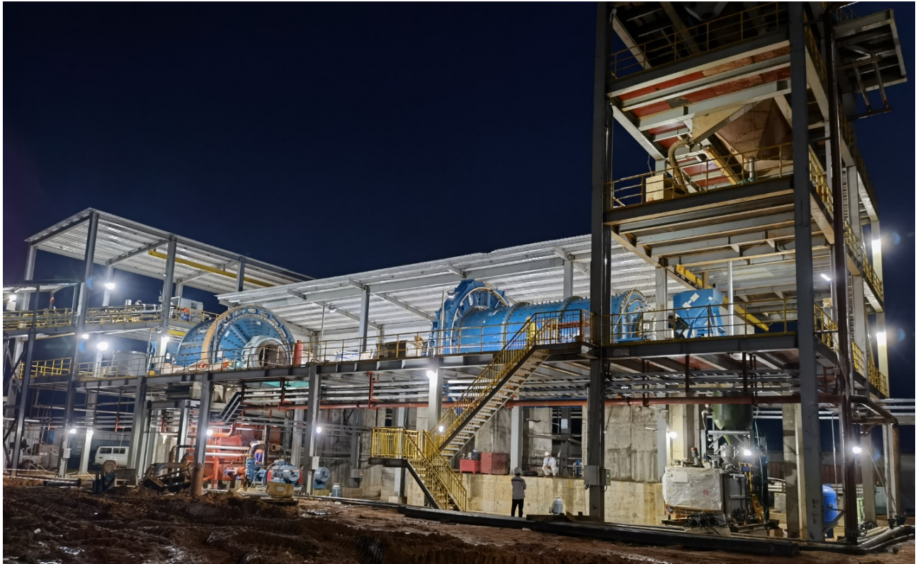
Figure 2: SAG & Ball Mills being commissioned
