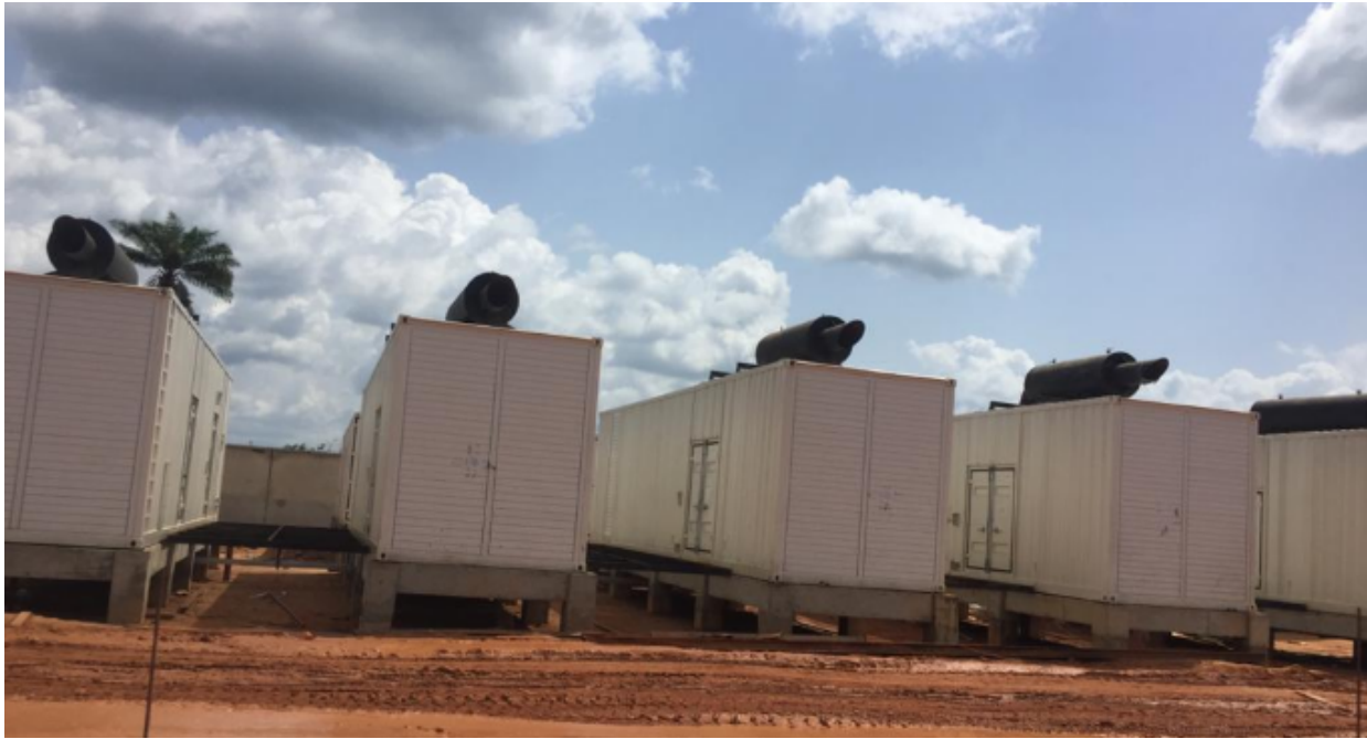
Figure 2: Power Generation Units installed
